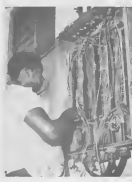
CABLES FROM crude tanks in receivers by Clinton Lynch, electrician here. A. CABLEMAN FOR of tankman den and sistema ta word mara na cableman for di receptoran door di Clinton Lynch.
